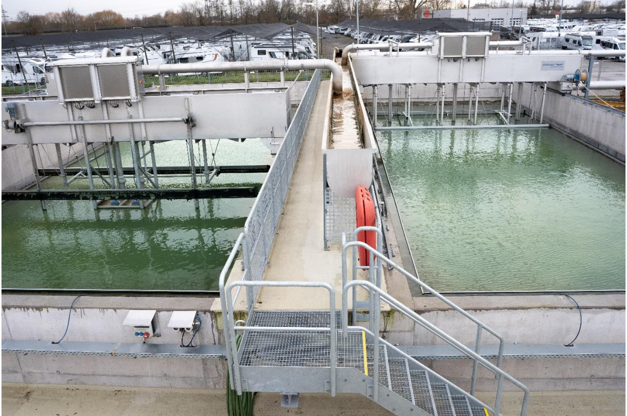
Figure: To ensure that all production water can be treated in-house at the Kehl site, new tanks and sand filter systems were installed. Source: Koehler Group
