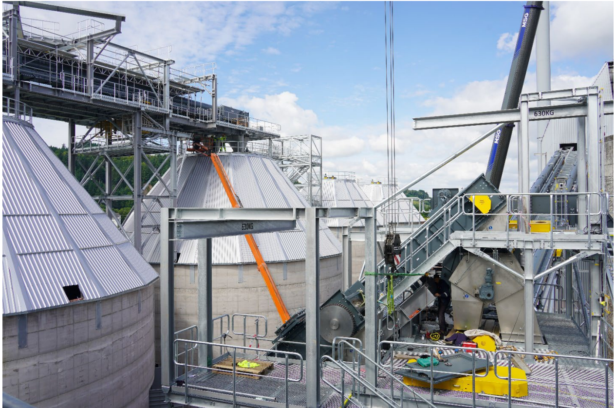
Figure 2: The conversion work on the heating plant continues to progress. Quelle: Koehler-Gruppe
